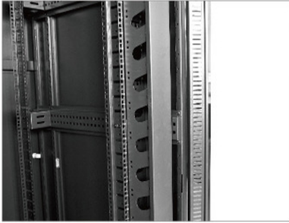
• Vertical cable management
