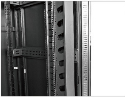
• Vertical cable management
