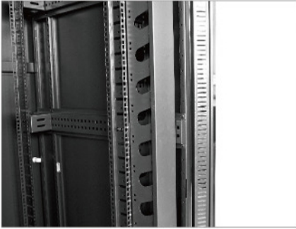
• Vertical cable management
